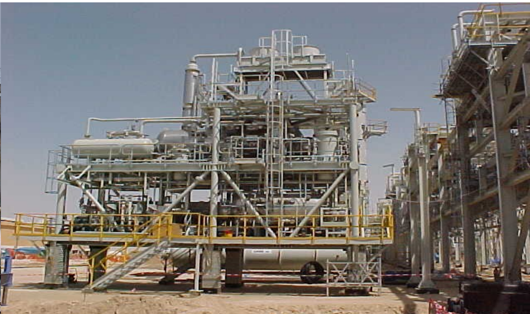
GLYCOL REGENERATION UNIT
